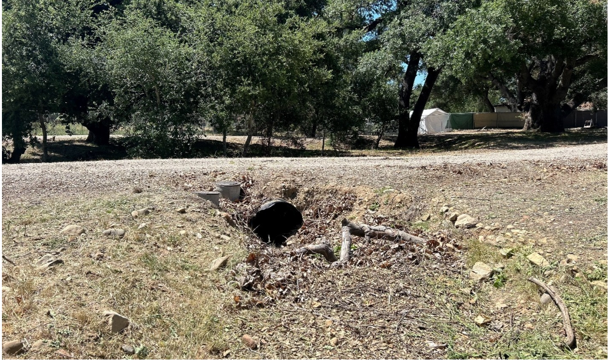
Photograph 13. View of road culvert at OWS Wellfield laydown yard (west of San Antonio Creek), facing south.
