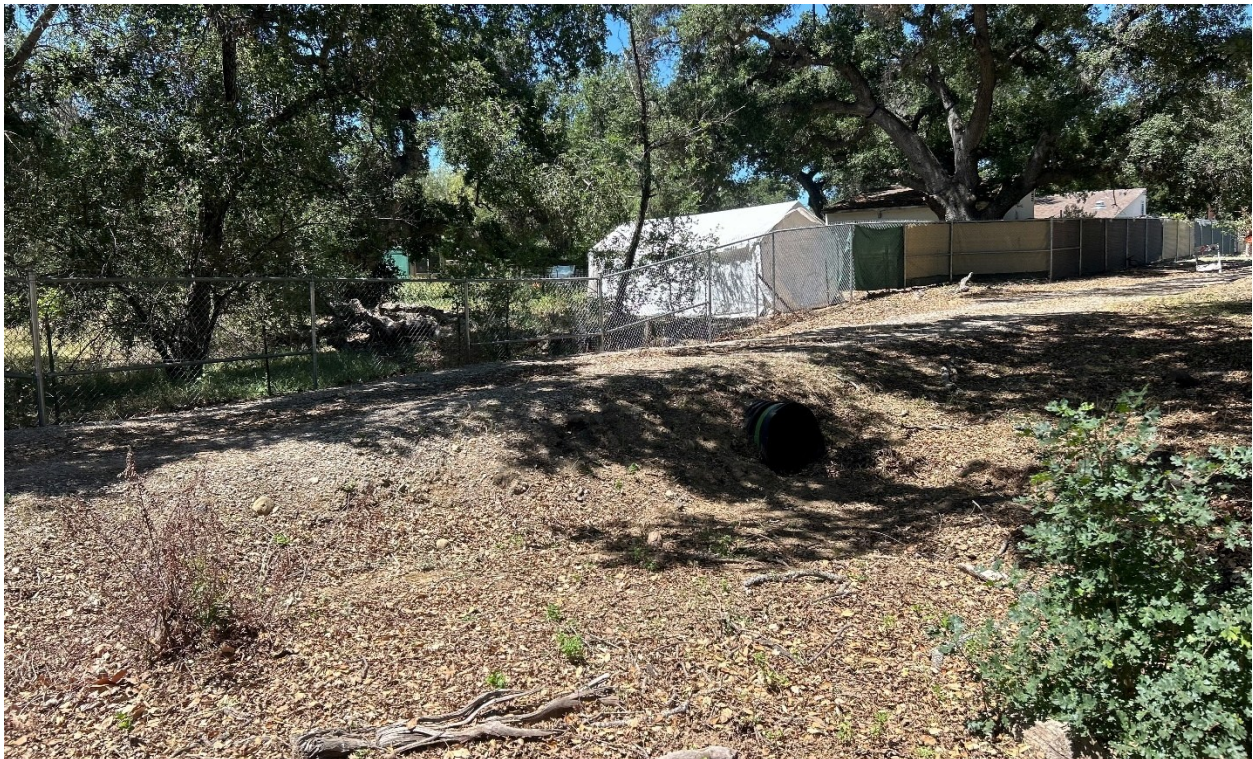
Photograph 14. View of additional road culvert at OWS Wellfield laydown yard (west of San Antonio Creek), facing south.
