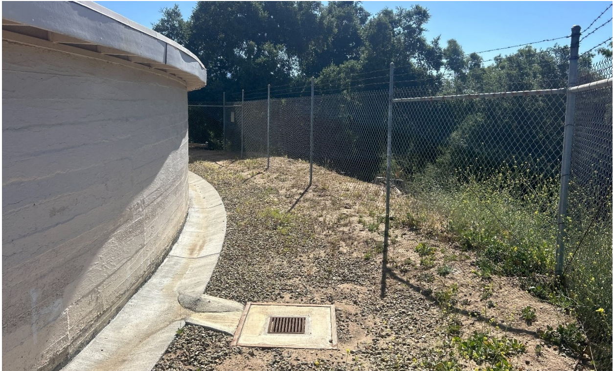
Photograph 7. View of existing Arbolada Tank and Pump station site with drainage system, facing east.
